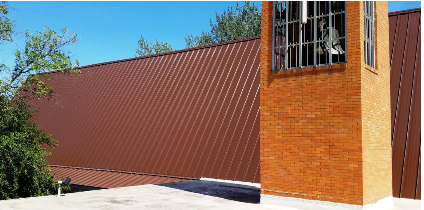
Top picture - West side roof after; Bottom - View from front of church
